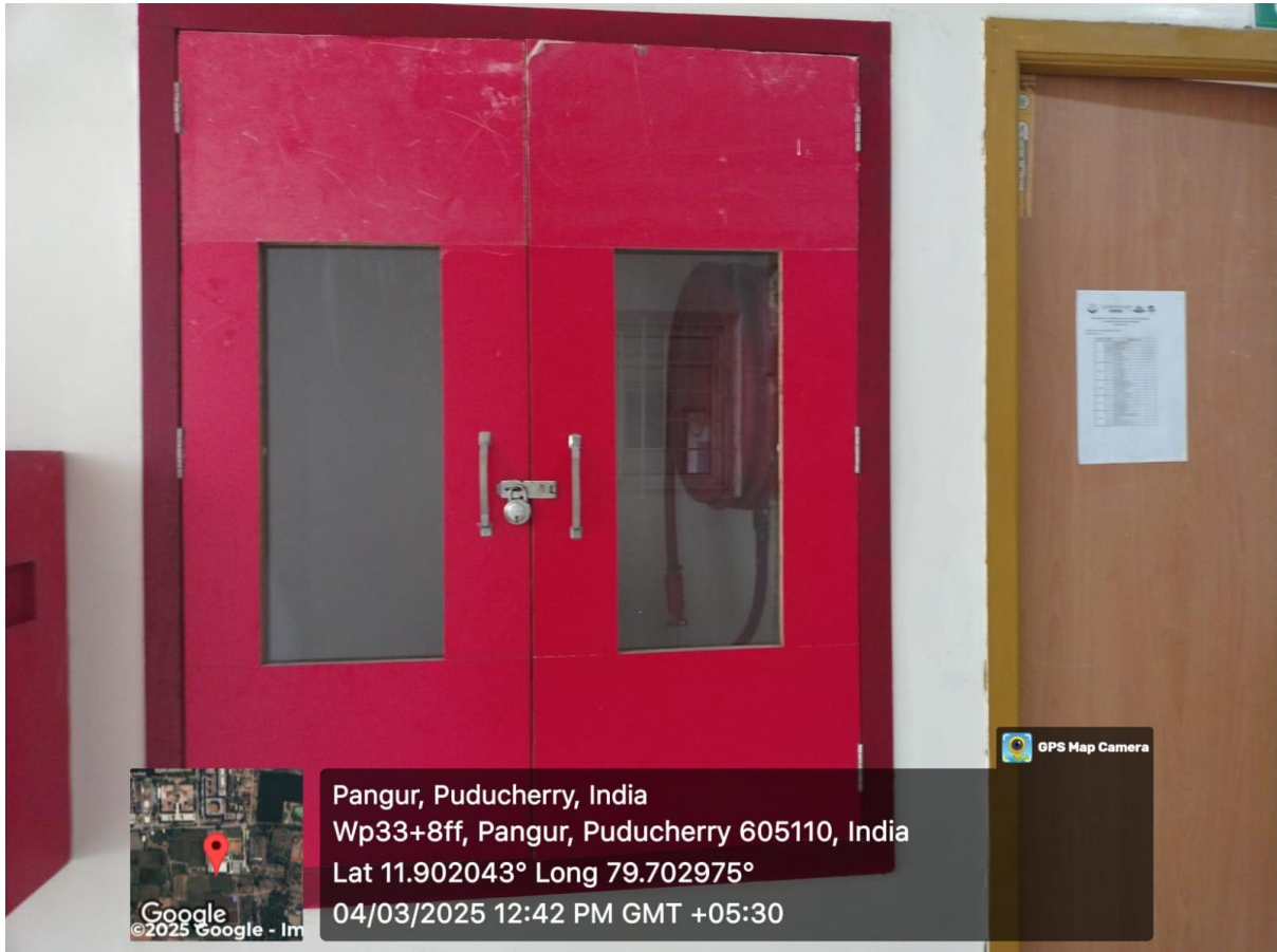
Figure ii: Fire Safety Alarm
